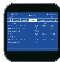
UPS Cabinet Control Panel
